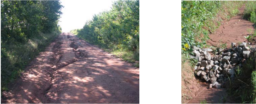
Figure 3. Clay roads are prone to erosion and check dams must be cleaned regularly.
